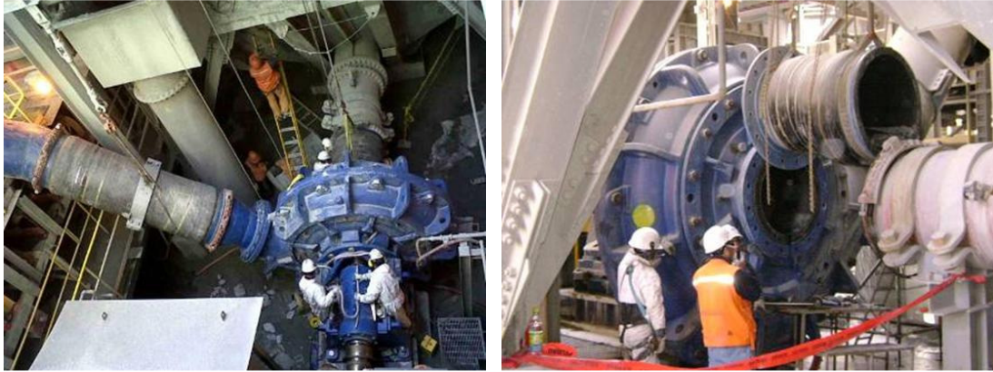
Figure 29 – Suction with Expansion Joint and Discharge with Hose
