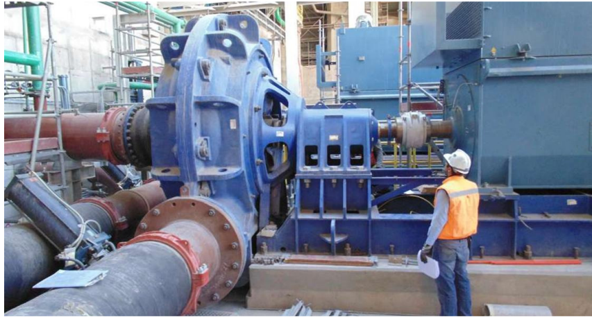
Figure 38 – Mill Circuit Pumps, maintenance interferences
