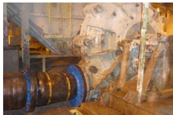
Figure 28 – Expansion Joint and Hose
